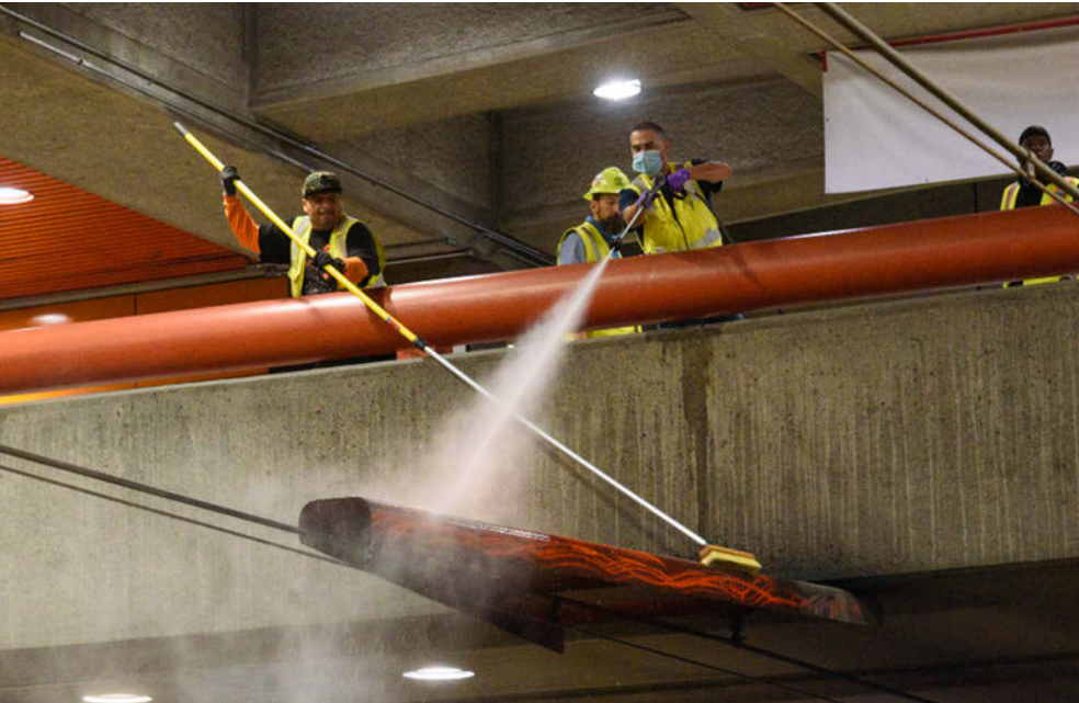
Track crew power washing and removing trash from trackway during Fix It Week night maintenance work.
