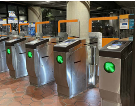
WMATA's 55-inch fare gates installed at Fort Totten Station.
