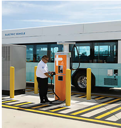
The ChargePoint Express Plus DC fast station in use.
