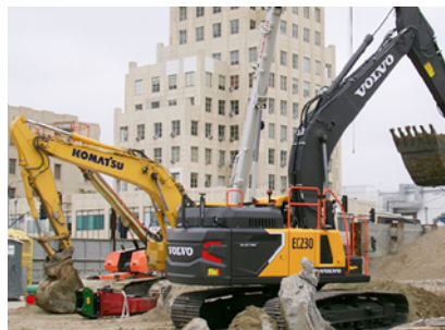
Skanska is piloting a zero-emissions electric excavator on L.A. Metro's D Line Extension Transit Project.
