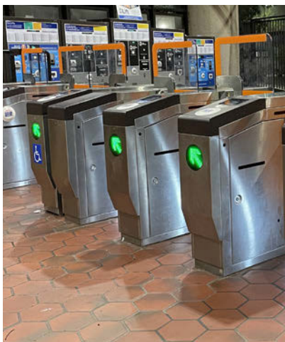
WMATA will retrofit its Metrorail faregates with a new design aimed at combating fare evasion. Photo: WMATA
