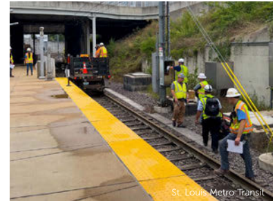
ST. LOUIS Metro Transit crews working to repair infrastructure damaged by flooding from an end of July storm.
