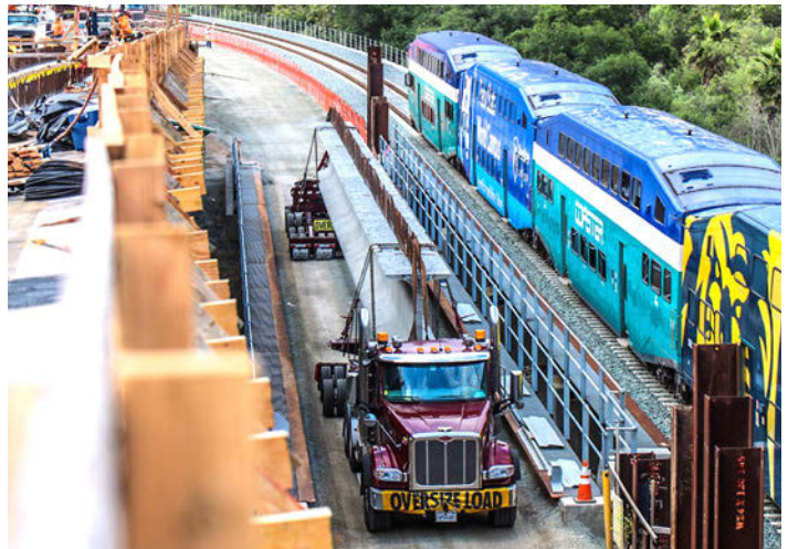
MCTC WORKED closely with NCTD to ensure certain construction activities could continue adjacent to active tracks.
