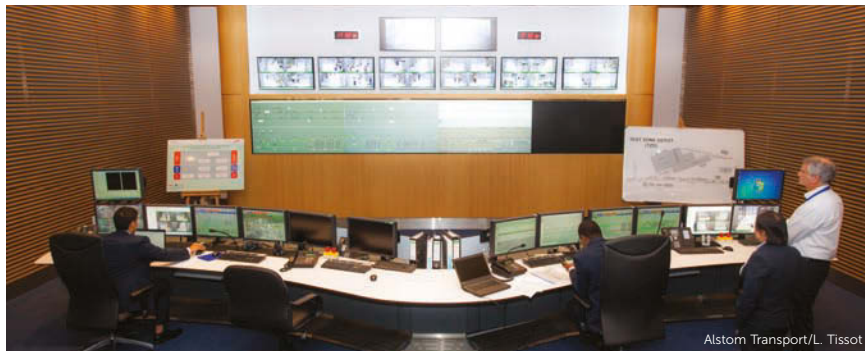
THE OPERATION control center includes automatic train supervision and SCADA, security surveillance monitors, AVLS and a police control room.
