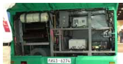
The electrical equipment on the LiAZ bus was in a full height compartment at the rear.
